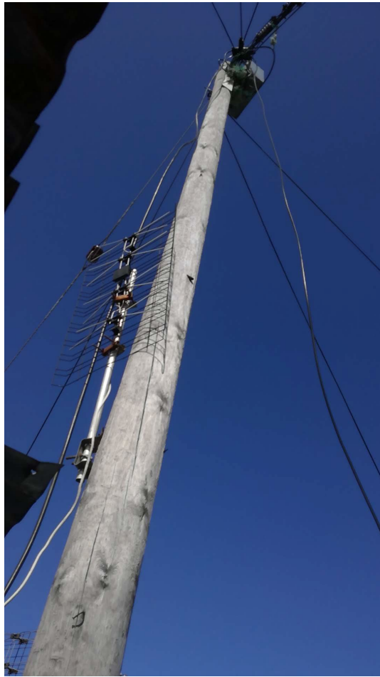
FIGURE 21 Electrical spiderwebs [Altamore S, 2019]
