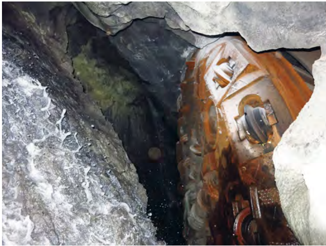
Fig. 1 Cutterhead of a tunnel boring machine inside a large karst void with a discharge of several \text{m}^3/\text{s} . The drive came to a standstill for several months and discharge from the spring related to of the karst conduit network was impaired.
