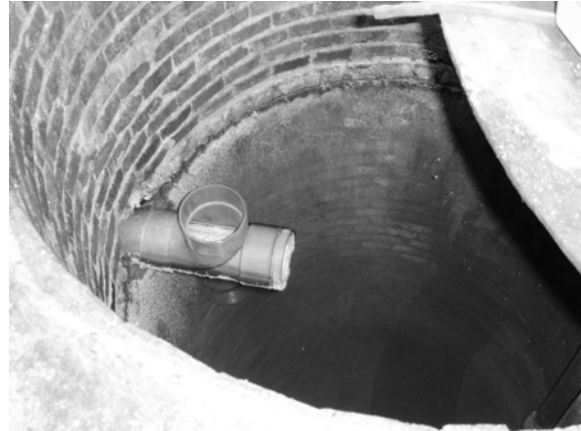
Figure 8.7: View of the Gontard well head (July 2008).
