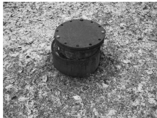
Figure 8.6: View of the F99 well head (February 2008).
