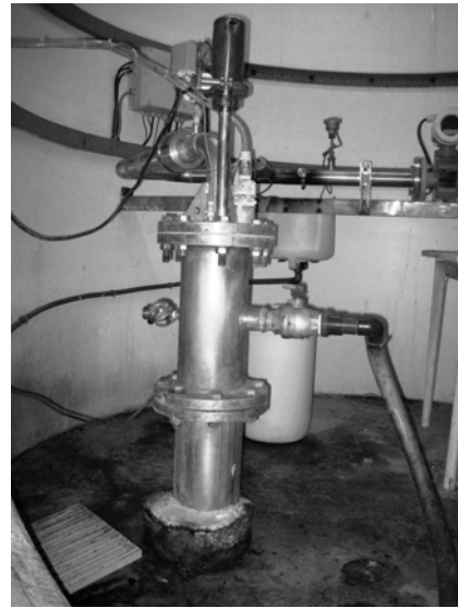
Figure 8.5: View of the De Mey Ouest well head (February 2009).
