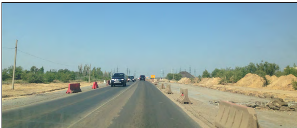
Figure 33: Volgograd Aviators' Highway under construction in 2016. At this point the expanded lanes had not yet been opened for use, but the newly repaved parts of the road were already cracking.
