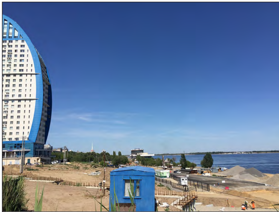
Figure 18: Construction of the new prodolnaya , or parallel road, along the banks of the Volga River about 5km south of Volgograd’s World Cup stadium, next to a pair of elite apartment buildings.
