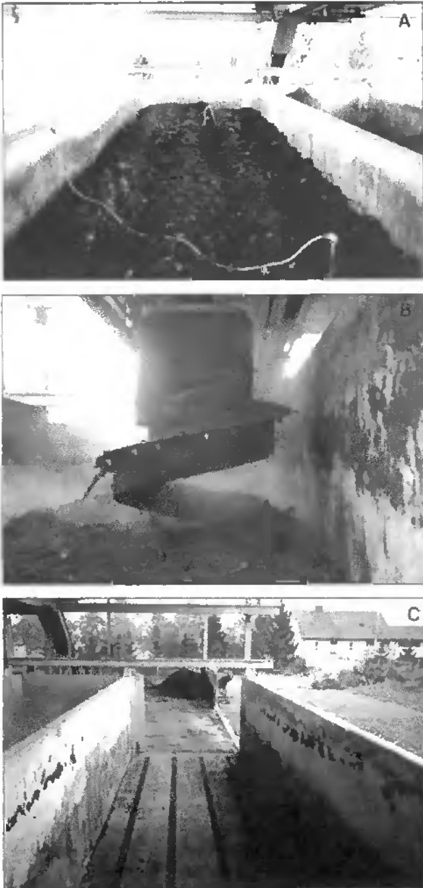
Figure 51: Temperature probes (A), turning system (B), and aeration channels (C) of the box composting system.
