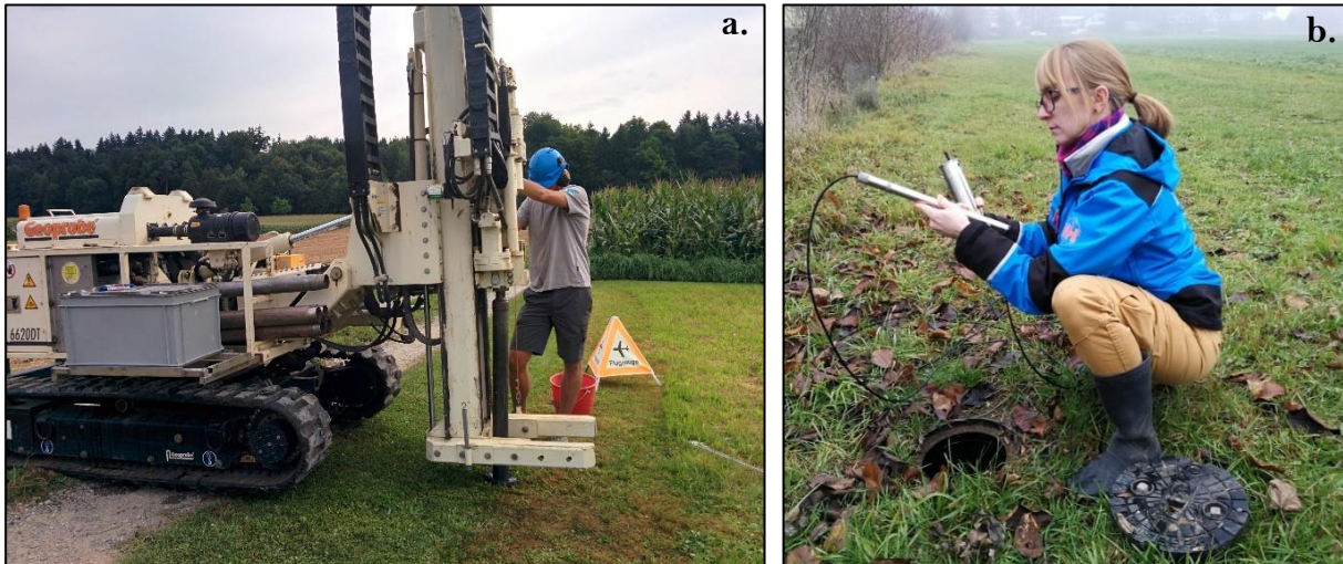
Figure 1-1. Groundwater monitoring wells allow us to directly observe and sample the subsurface. a.) installation of monitoring wells and soil core collection with a direct-push Geoprobe; b.) wireless sensors allowing for continual monitoring of basic groundwater conditions.
