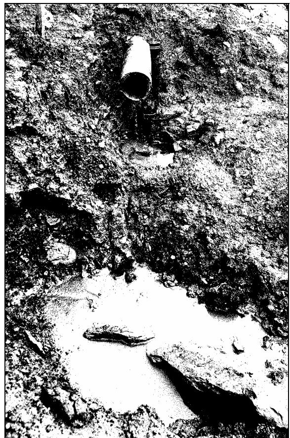
Figure 6. Photo of the broken water pipe where it intersected the western side scarp of the slide body.
