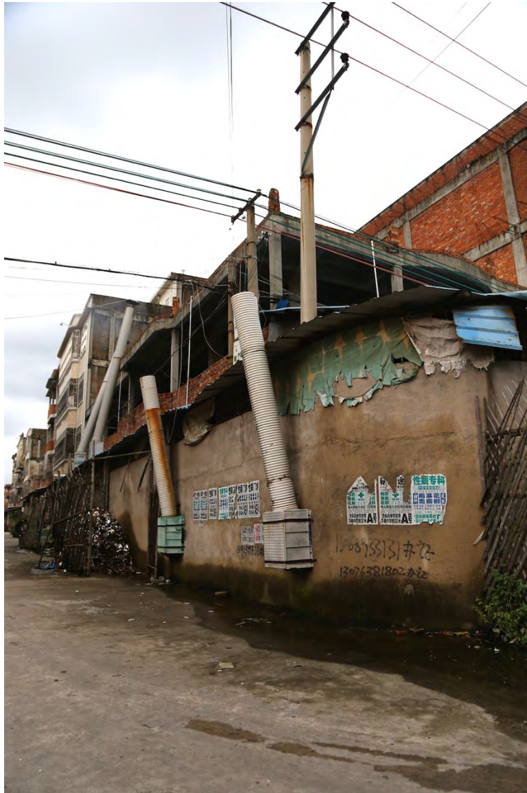
Figure 4.6: Exhaust fans and air ducts in Guiyu in the mid-2010s. Photo credit: the author.
