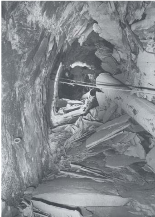
Fig. 1. Slabbing at 2600m depth in a quartzite [15] due to long axial tensile cracks propagating at low confinement near the excavation boundary. This is analogous to axial splitting of unconfined or lightly confined compression tests.
