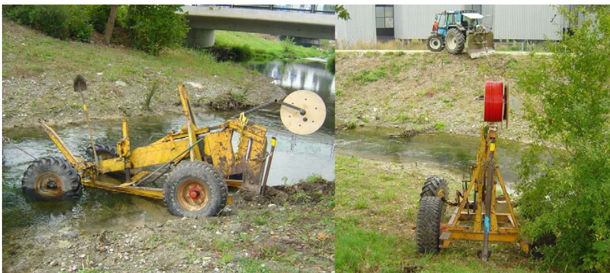
Figure 4.2. Tractor-pulled plough employed for the installation of the fibre-optic cable in the streambed of the Chriesbach.
