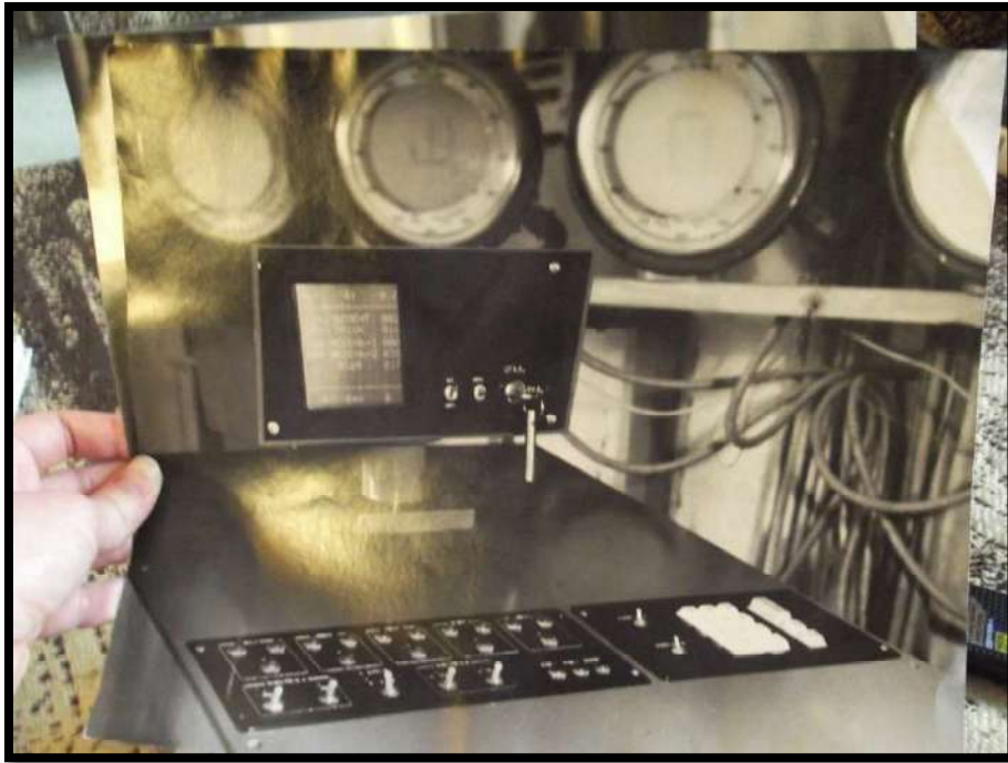
Figure 34. Photo of a self-made computer installed in the workshop of a concrete batching plant From Yurii's home archive. Photo: Zinaida Vasilyeva
