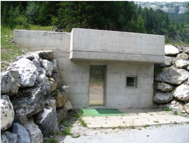
(a) Structure that drains about 10% of total spring discharge, where the community of Conthey collects fresh water.
